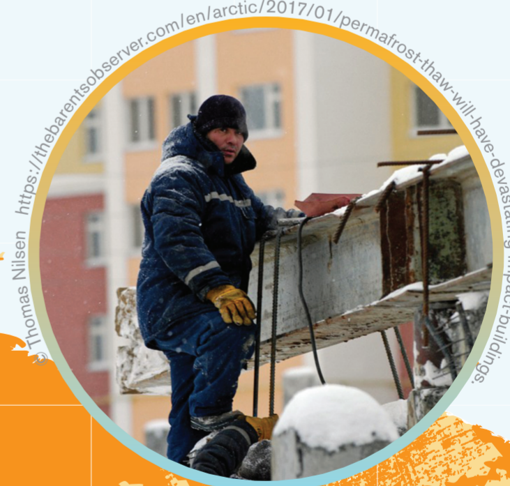
One solution has been to insert metal pipes along the perimeter of buildings to freeze the soil in the summer and maintain stability.
